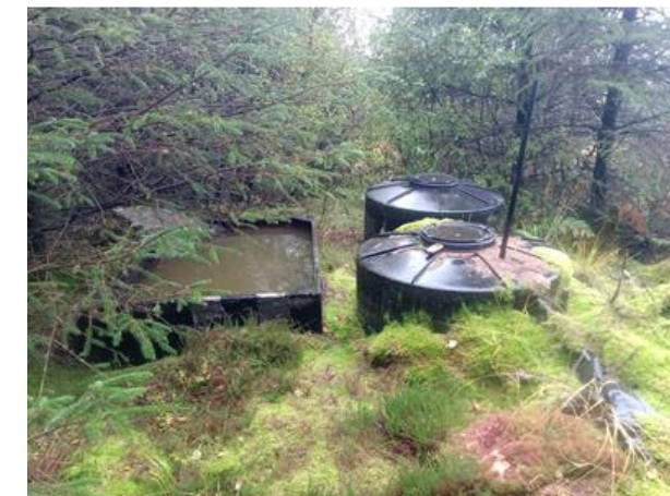
Photo Insert 8.6: PWS Infrastructure at Holmshaw
