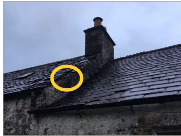
Photo 2: Re-entry point in crevice between slates and stonework at the front of the house.
